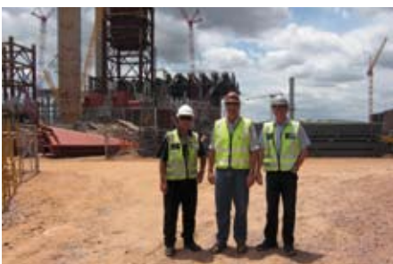
Ready to start the tour: (from left to right) Wayne Lamont (Site Manager), Jaco van der Westhuizen (Managing Director CBZ), Franz Bartels (President & CEO Clyde Bergemann Power Group)
